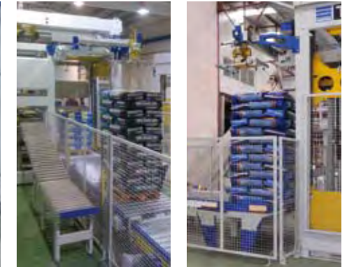
Automatic bags check-weighing and rejection
